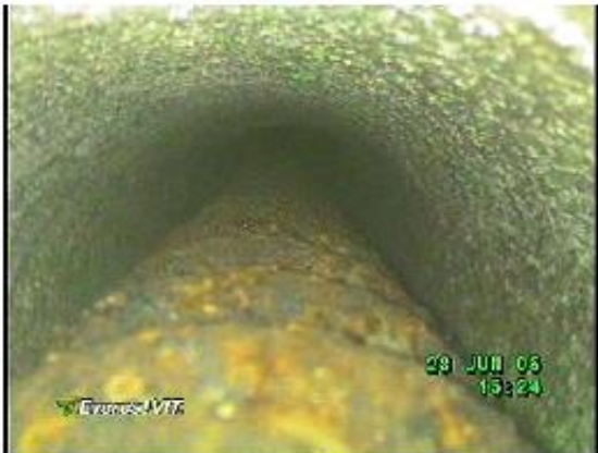
Void in Pier With Dywidag Bar Instead of Tendons
