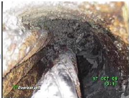
View of Void Bottom Corrosion on Duct and Tendons
