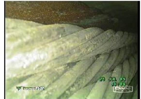
Corrosion on Duct
