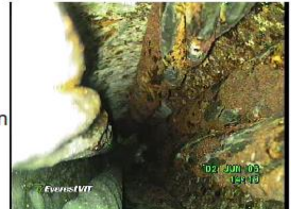
Corrosion on Both Duct and Tendon
