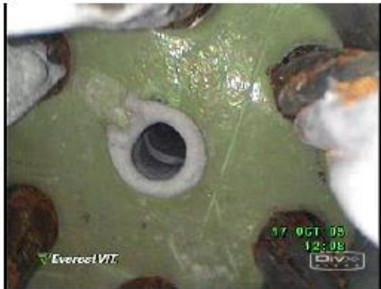
Close-up of Anchor. Top of Tendons Show some Corrosion
